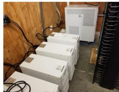
Fig.4.6 Battery Back Up System
